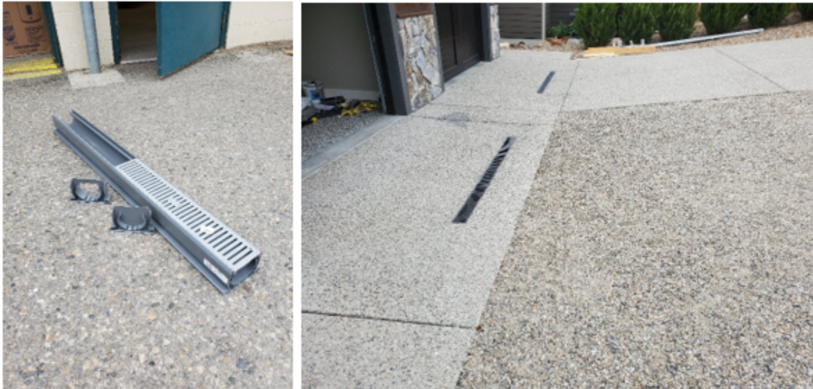
Figure 5 Driveway area catch basins
