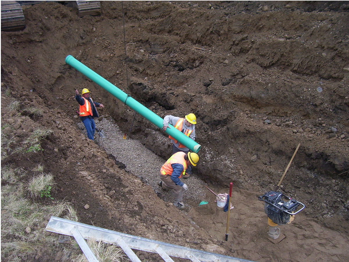
Figure 12 PVC gravity sewer piping at substantial depth
