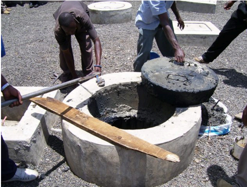
Figure 2 Manhole lid and cover
