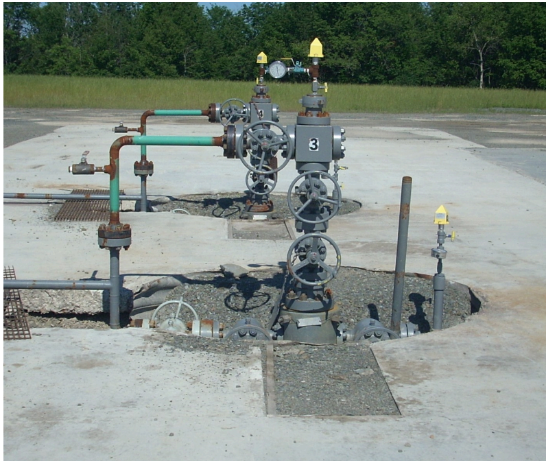
Figure 2. Gas well head Christmas tree.
