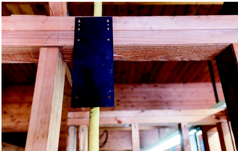
Figure 17 Striker plate protecting CSST tubing
