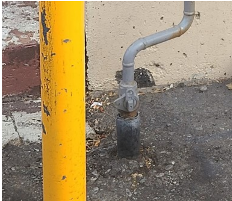
Figure 19 Sleeved gas service pipe
