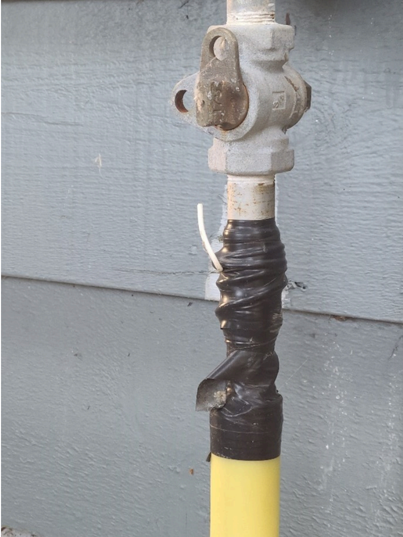
Figure 21 PE Sleeved meter riser with tracer wire for PE tracing
