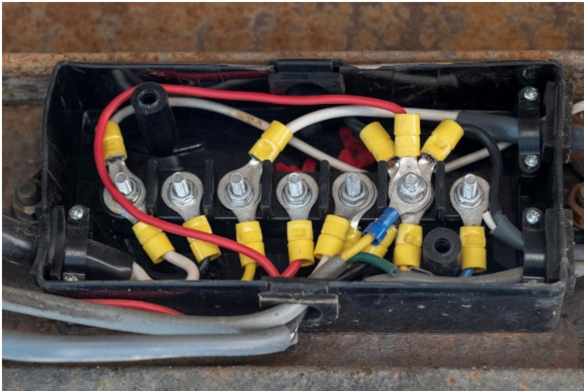
Figure 8 Sealed junction box using terminal posts (studs)
