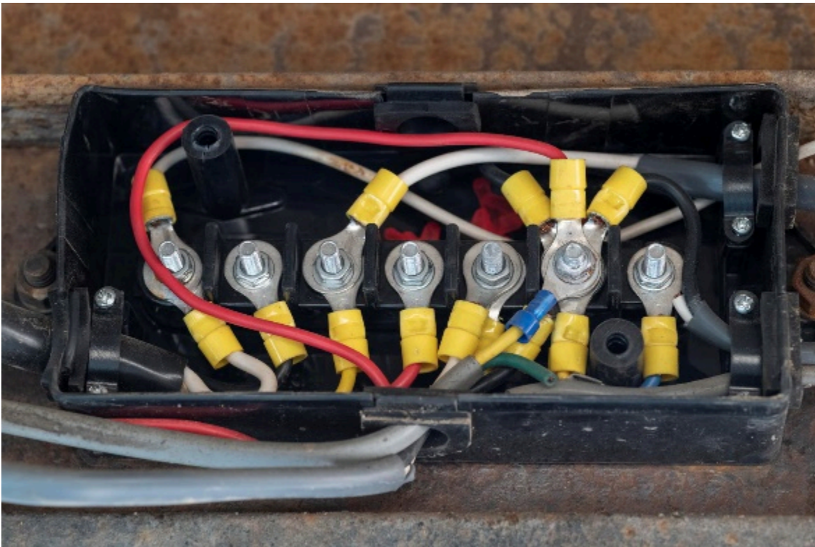
Figure 8 Sealed junction box using terminal posts (studs)
