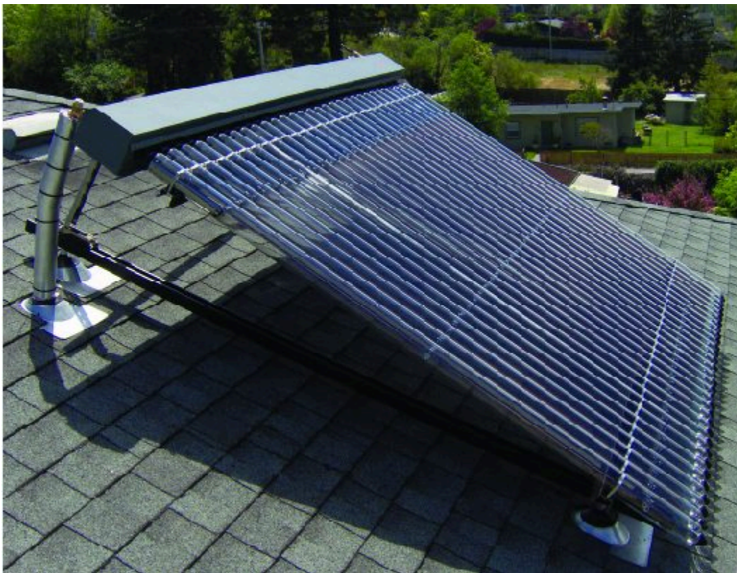
Figure 4 Evacuated tube collector in position
