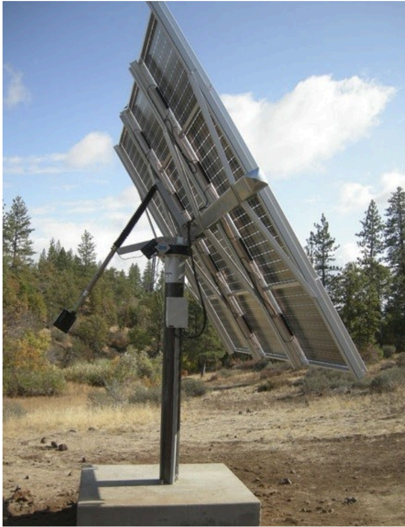
Figure 3 Pedestal-mounted PV array
