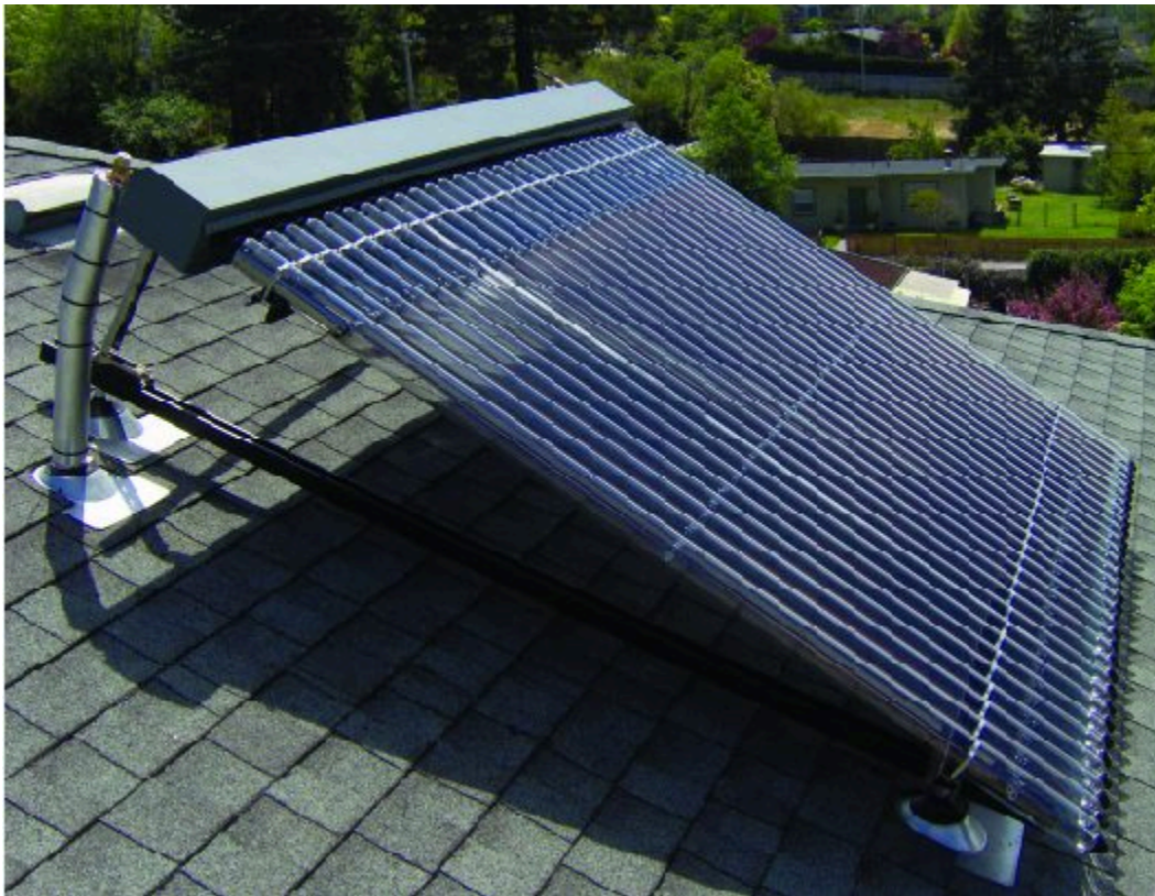
Figure 4 Evacuated tube collector in position
