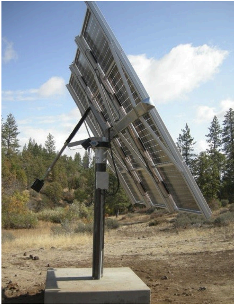
Figure 3 Pedestal-mounted PV array
