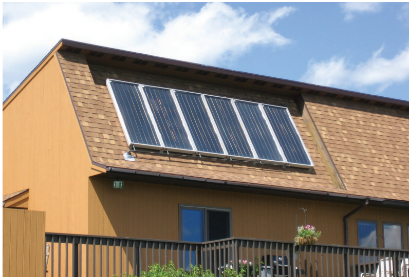
Figure 4 Roof slope increased to accommodate optimum solar angle for collector array
