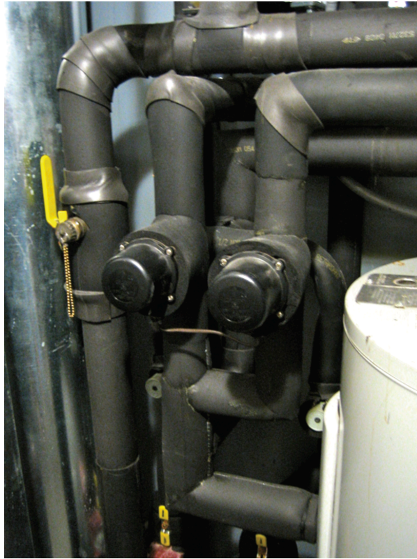
Figure 2 Insulated piping and fittings
