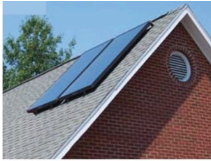
Roof-mounted flat plate collectors
