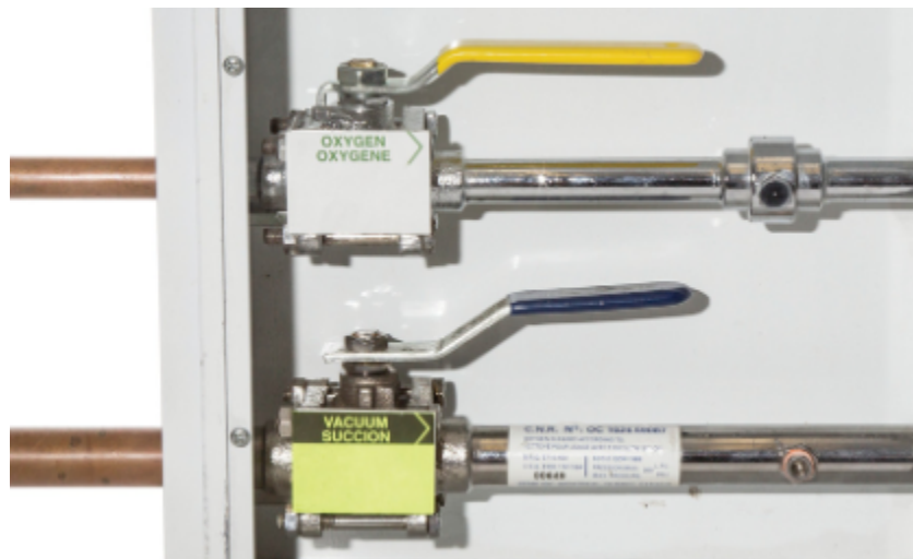
Figure 36. Labels for zone valve control box
