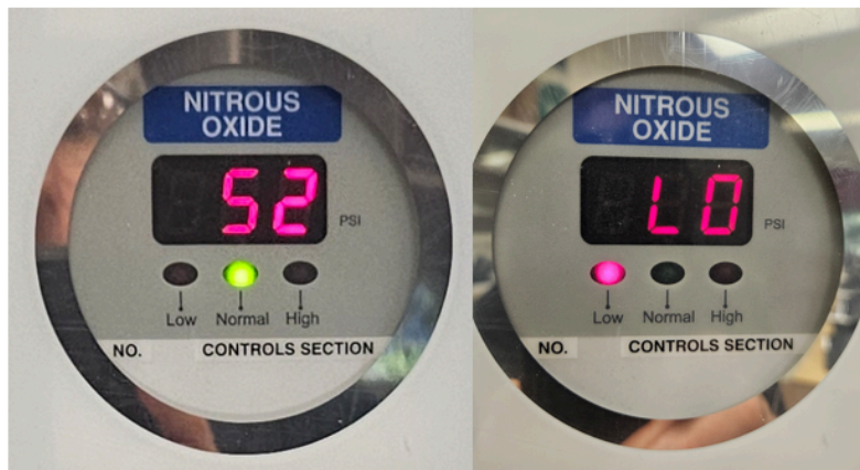
Figure 6. Zone alarm pressure display
