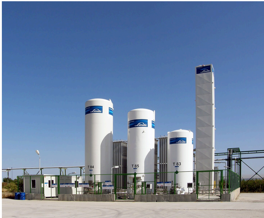
Figure 2. Bulk oxygen storage system
