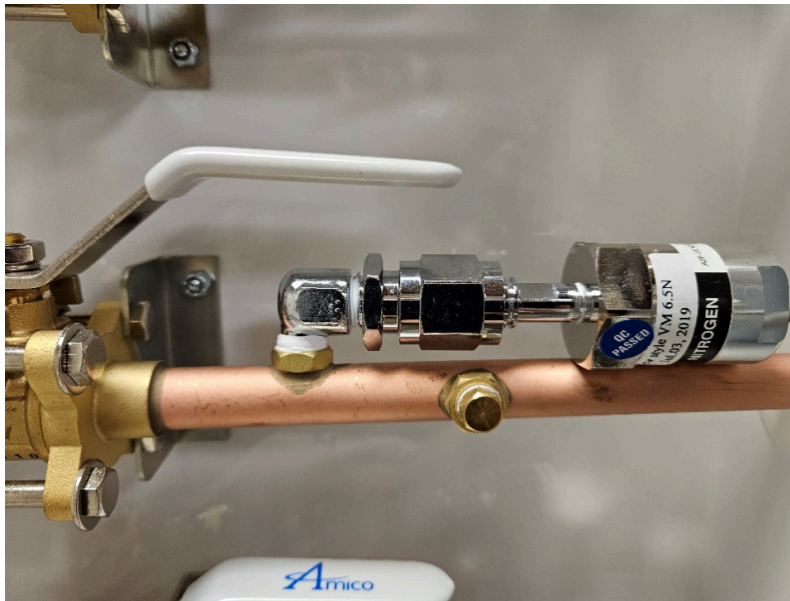
Figure 7. Gas specific pressure sensor assembly
