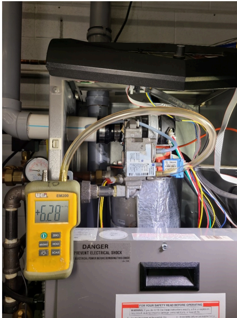
Figure 6. Checking appliance control valve inlet pressure
