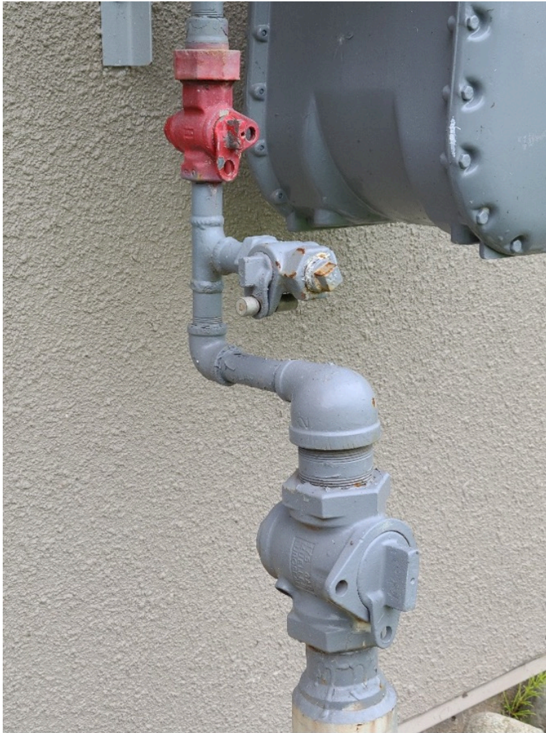
Figure 10. Luboseal™ gas valves on meter set supply
