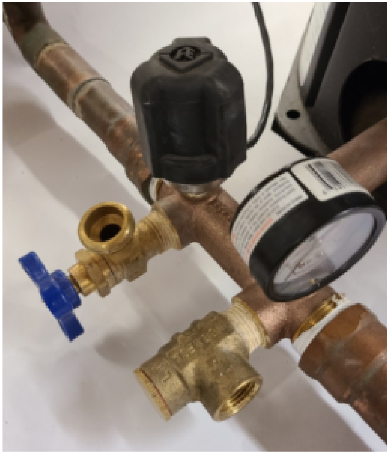
Figure 28. VFD pressure sensor
