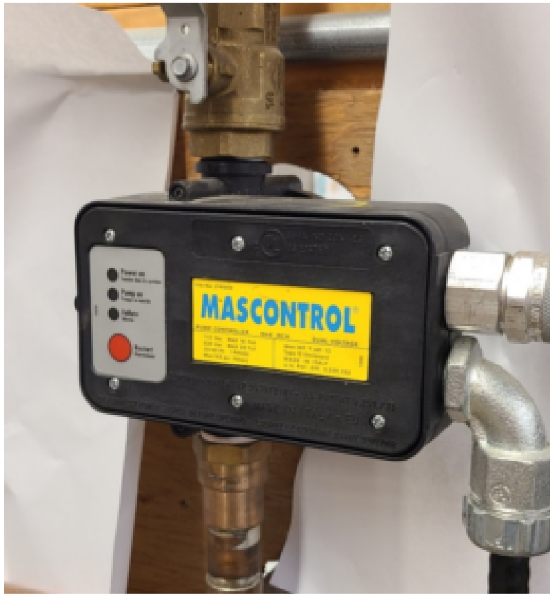
Figure 29. Mascontrol pump controller
