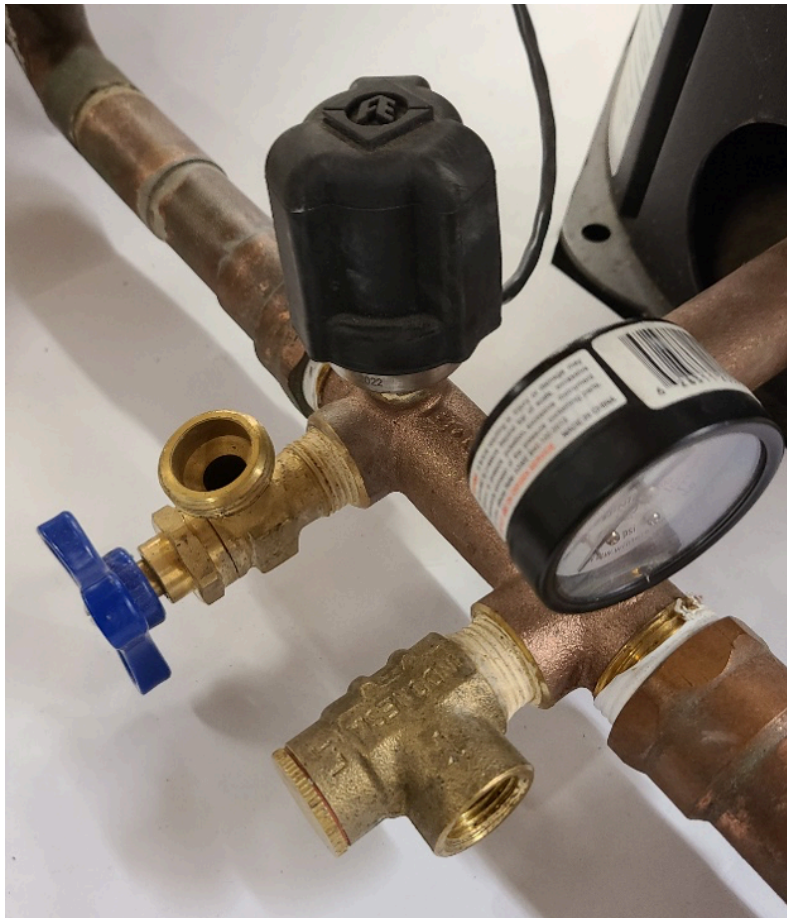
Figure 28. VFD pressure sensor
