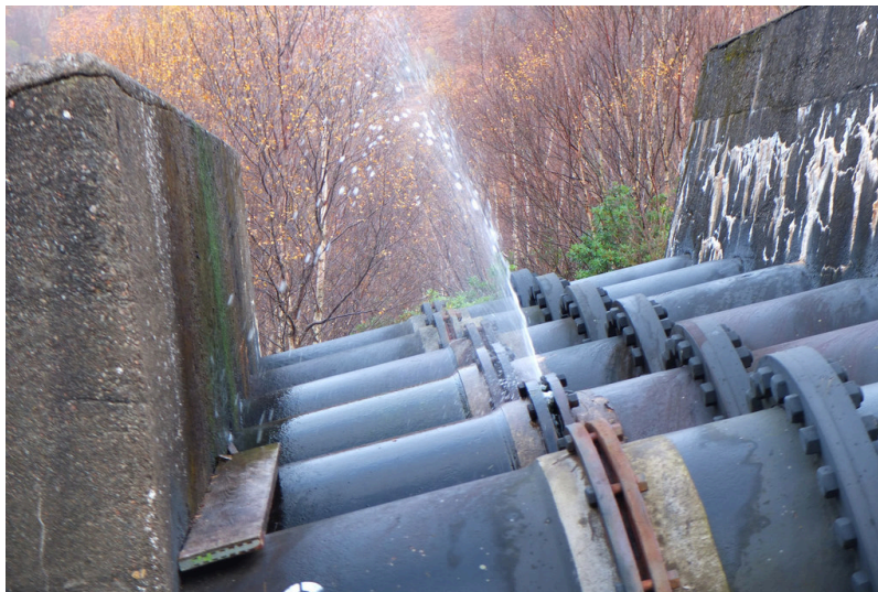
Figure 9. Water main break
