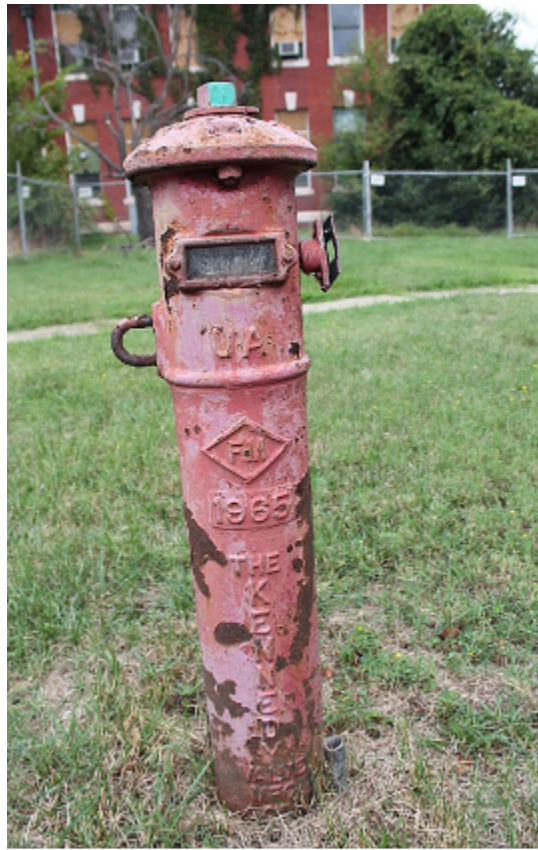
Figure 2. Post indicator valve
