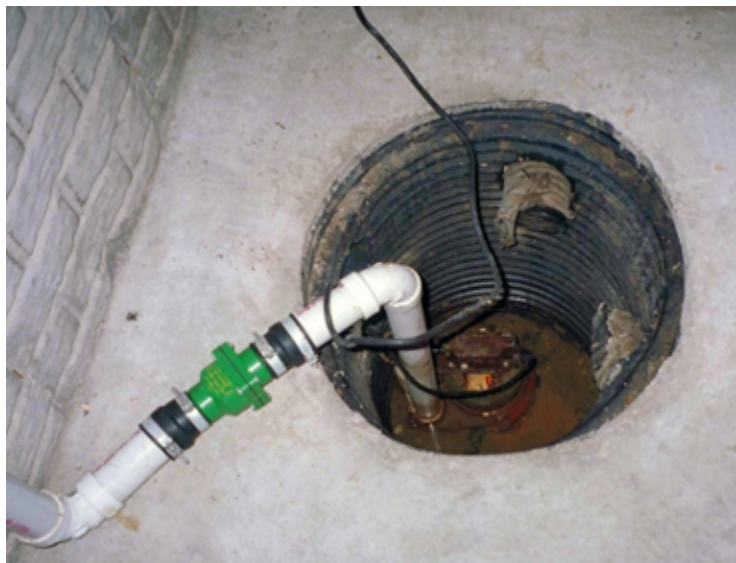
Figure 1. Basement Sump Pump
