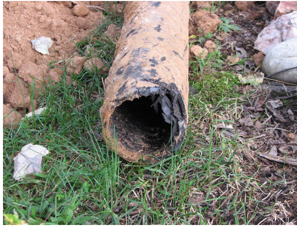
Figure 11. Corroded cast iron pipes
