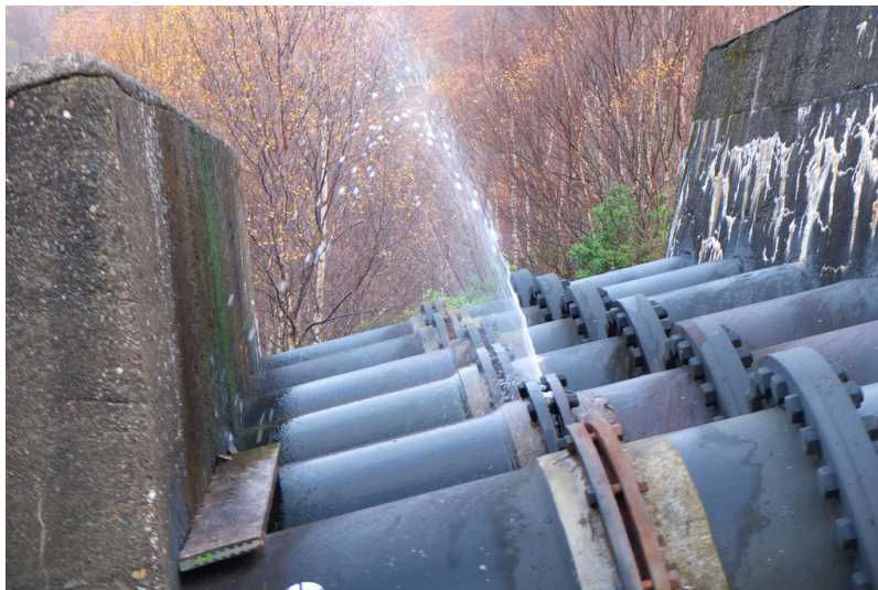
Figure 9. Water main break
