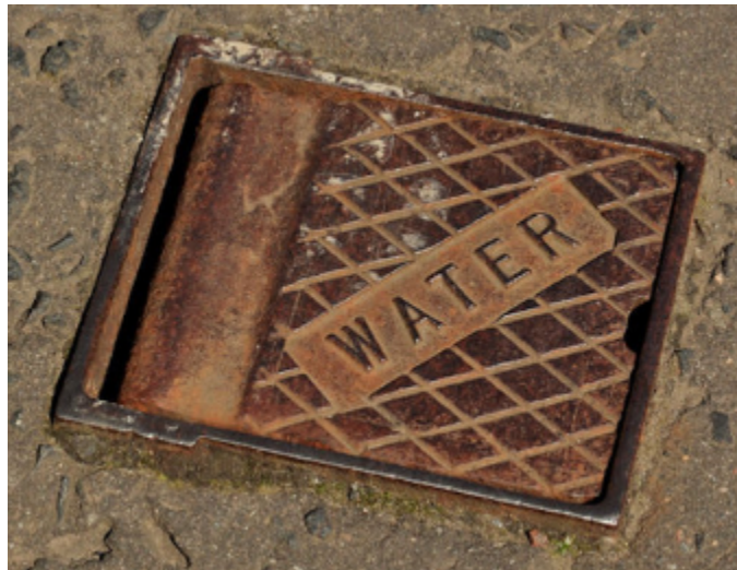
Figure 7. Curb stop valve cover
